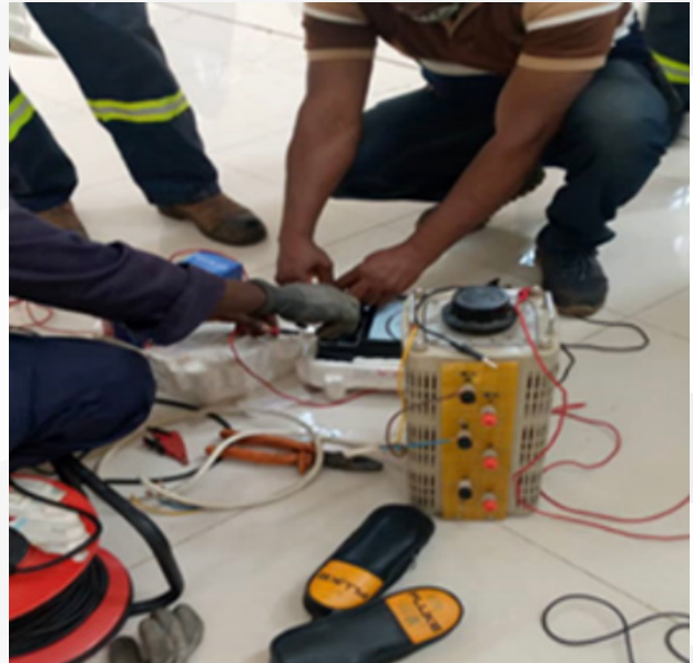
Figure 12: Conducting rotor pole drop test
