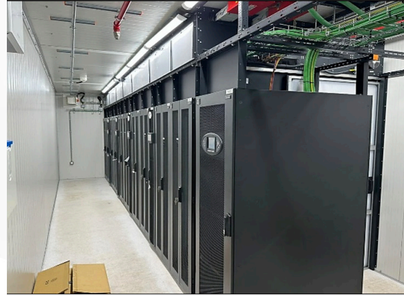
Figure 24: Internal view of modular datacenter
